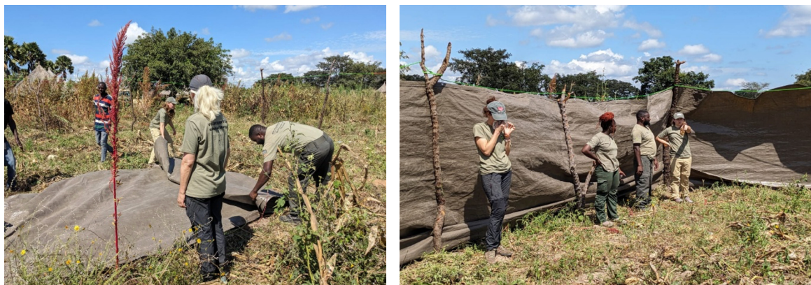
Figure 6: GRI team constructing a kraal for a community member from the phase 2 parametric drought insurance payout
